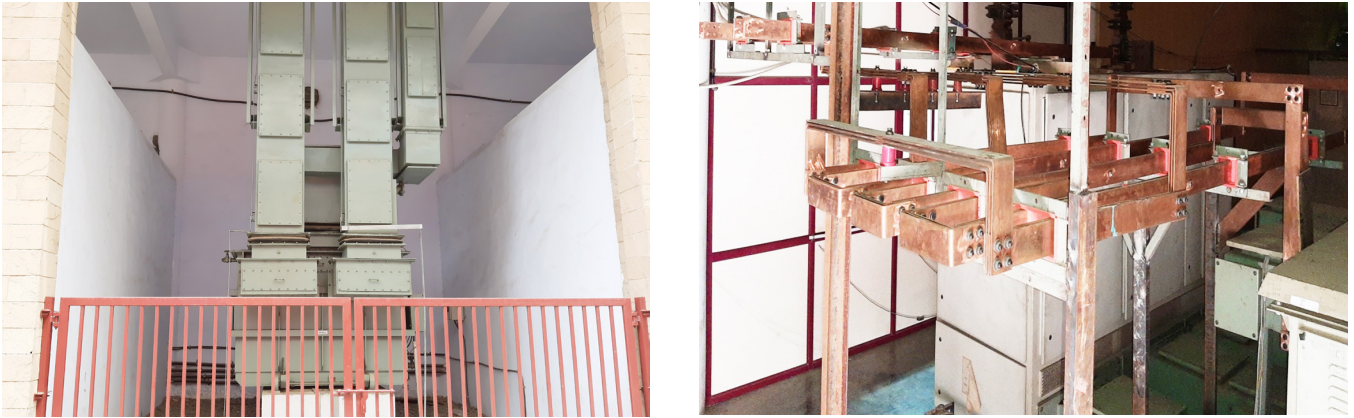
Figure A.3.5 Power supply for the SST-1 Poloidal Field (PF) coils have been commissioned Left - Transformer and Right - busbar connections to the PF coils inside the tokamak hall of SST-1
