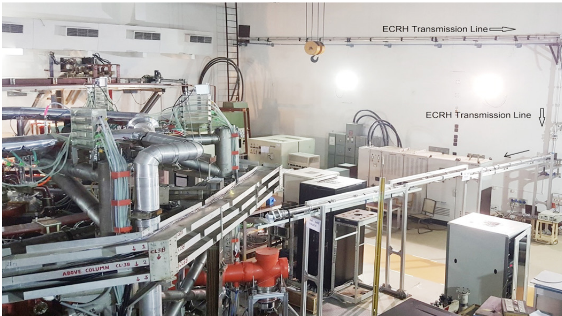
Figure A.3.3 ~75meter long transmission line is used to launch ECRH power from SST- hall to ADITYA-U tokamak, consisting of 63.5mm ID corrugated waveguide, bends, polarizer, DC breaks & bellows etc
